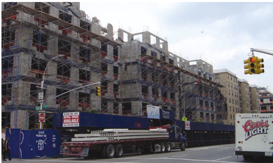
Construction is under way at 1955 First Avenue, which includes 231 apartments and 15,331 square footage of commercial space.
